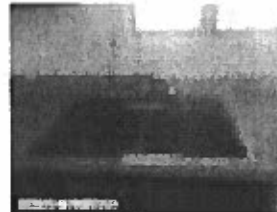
# 4989181344 Description: Condition Faucet Open - Condition Order Number: [REDACTED] CompletedDate: 4/7/2021
