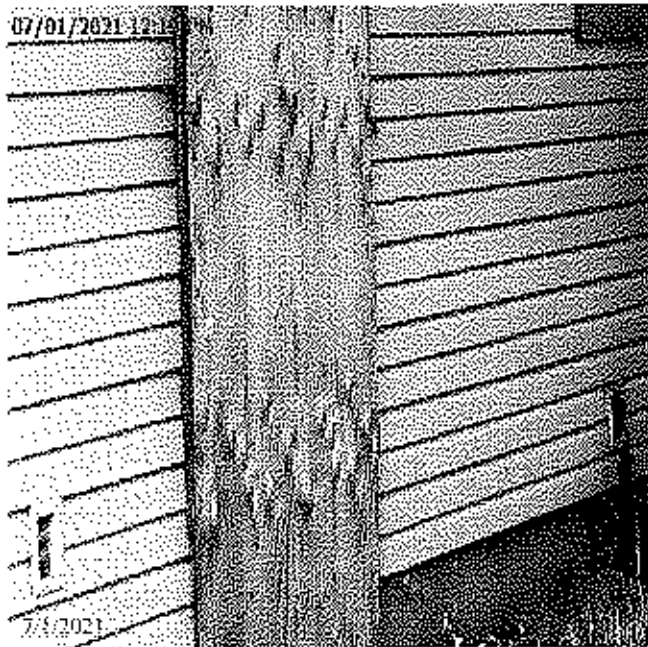
Address: 11312 NE DAVIS ST. PORTLAND OR 97220 Date Completed: 07/01/2021 Description: BOARDED DOOR
